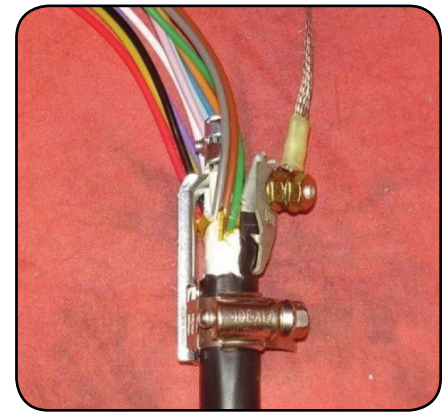
Bonding Clamp Installed
